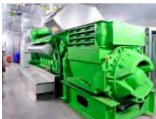
CHP engine protection
